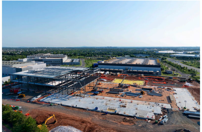
Gerville/iStock/Getty Images Plus construction of a data center in the United States
