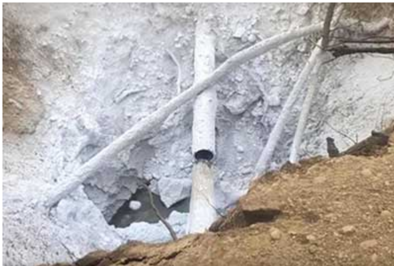
Ruptured pipeline in Satartia, Mississippi (The New American)
